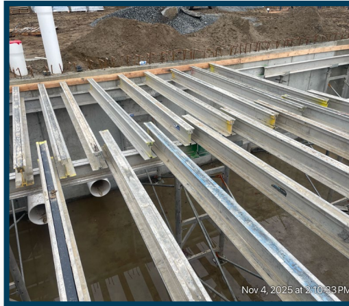
Form Surge Tank Lid
