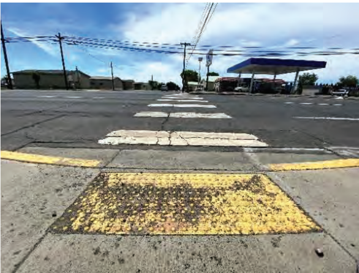
A crosswalk on SR 28 in need of repair.
